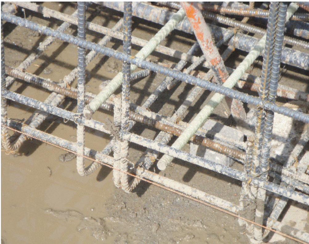
Rusted new rebar versus unruined GFRP form ties
